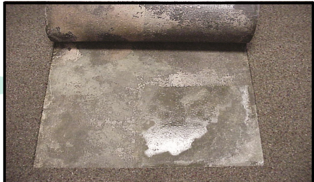
Moisture-related Floor Covering Failure (PCA image)
