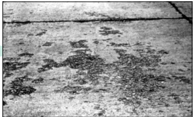
Scaling on Concrete Slab
