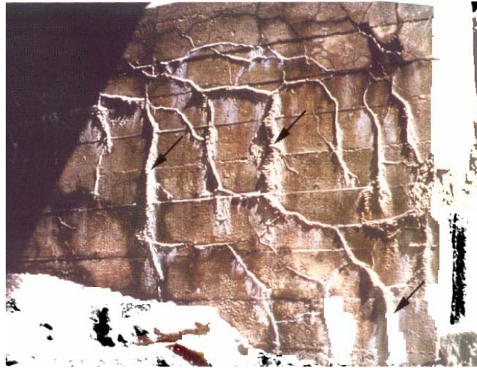
Figure 5. Cracking of a concrete bridge substructure due to ASR
