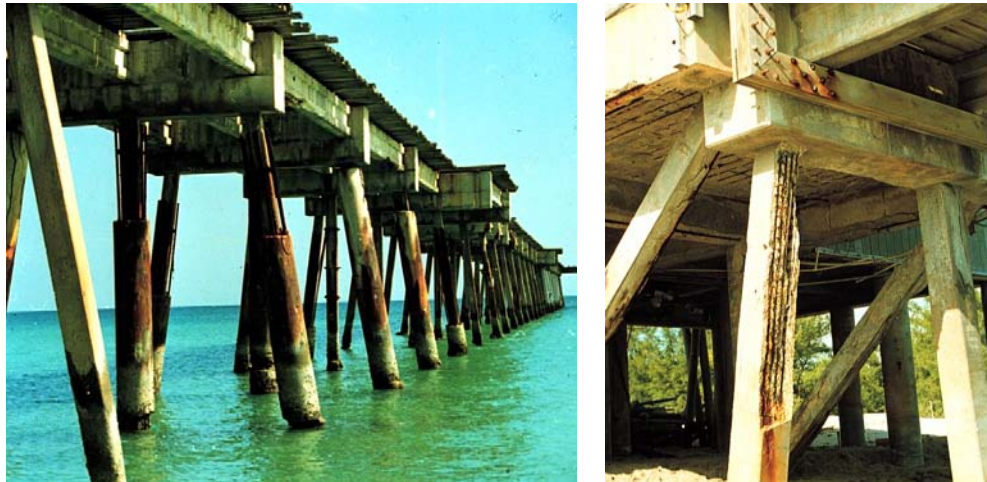
Figure 4. Corrosion of Steel Rebar Due to Chloride Ingress
