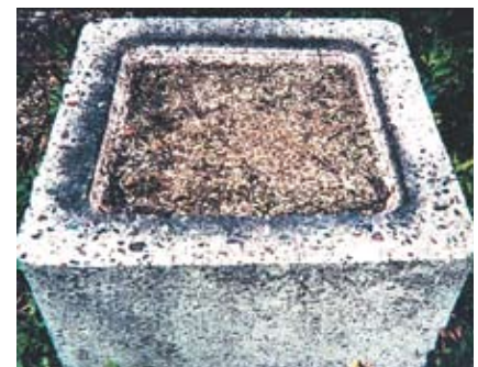
Figure 1: Damage due to exposure to freezing and thawing cycles. Courtesy Portland Cement Association.
