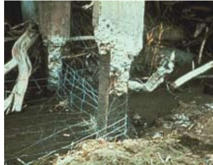
Figure 2: Example of deterioration of concrete due to exposure to sulfates.
