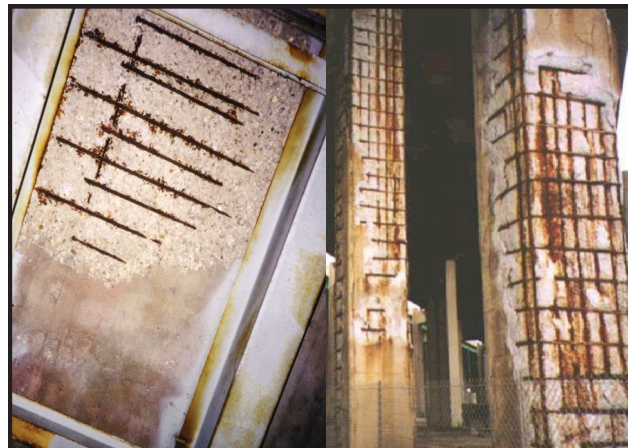
Reinforcement Corrosion in Structures
