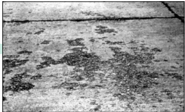
Scaling on Concrete Slab
